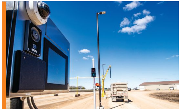
The facility operates like any other grain elevator for deliveries during regular business hours. After hours, RFID key cards, grain trailer ID tags, cameras and other automation systems enable grain delivery without staff present.
